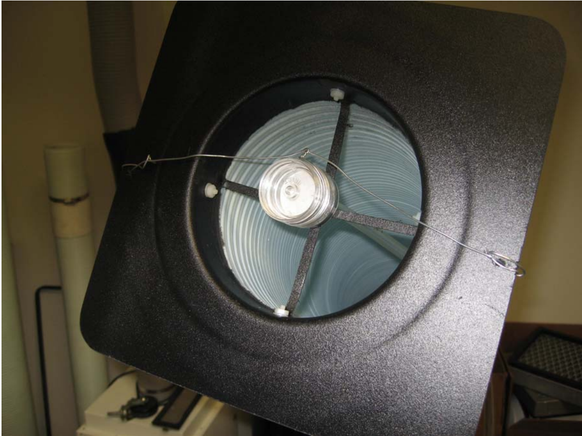
Photograph #3: The inlet duct of the welding fume extractor is shown above. The sampling filter cassette was wired in place to permit sampling of the air being drawn into the extractor.
